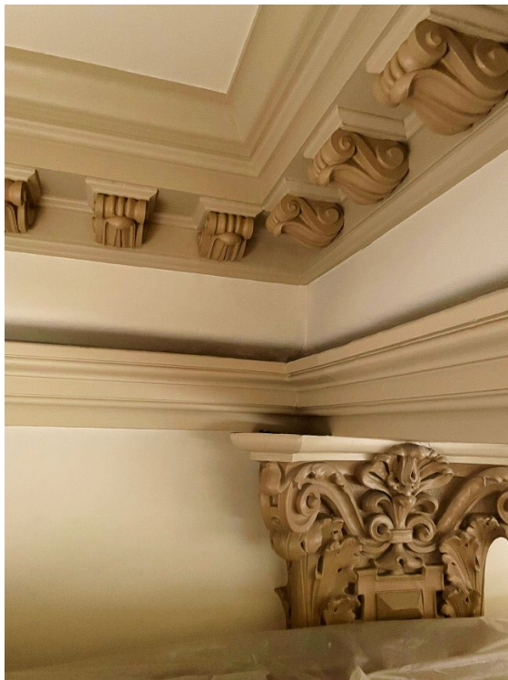
Sample of plaster detail in the ceiling and the multi-color paint scheme
